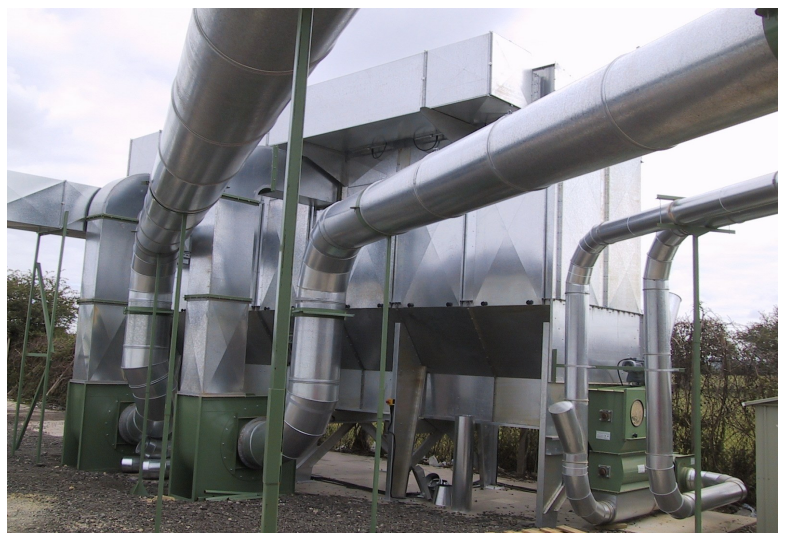
CHAINFILTER CH/6/4260/WP FEEDING BIOMASS HEATER
